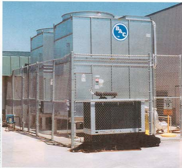
This cooling tower installation is operating at a public school in Arizona.
