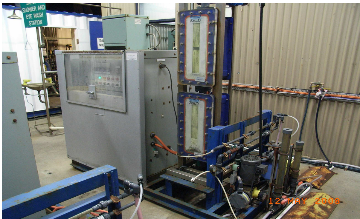
Figure No 10 – ElectroBrom 40 \text{ kg}\cdot\text{day}^{-1} Biocide Electrolysis Unit.
