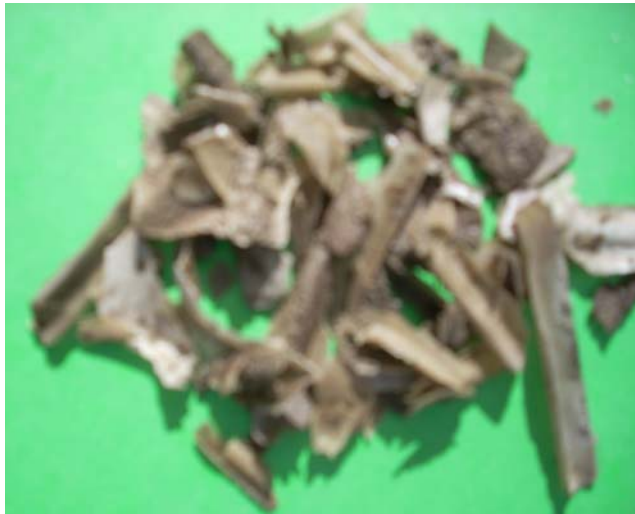
Scale Found in NCD Treated Cooling Tower
