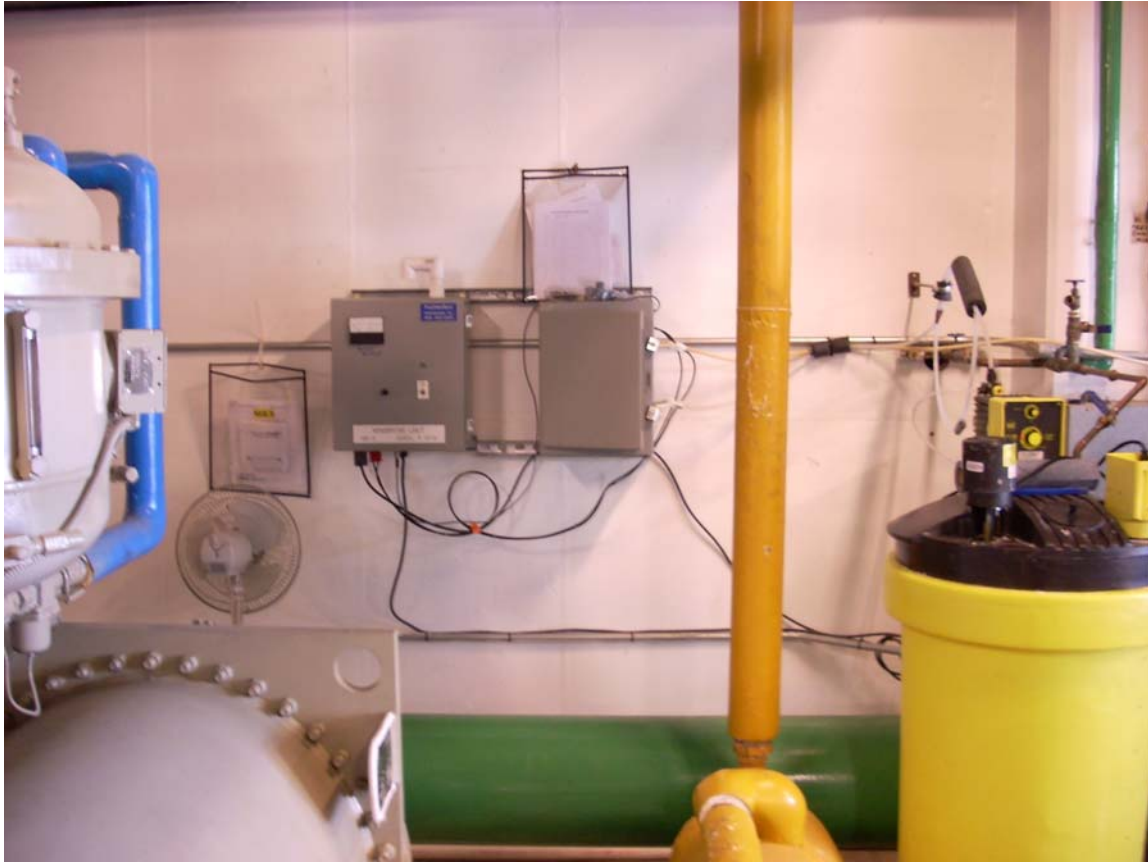
Former steel cell housing MiniBrom Model MB 5 installed in major hospital power house Yellow plastic dilution tank to the right
