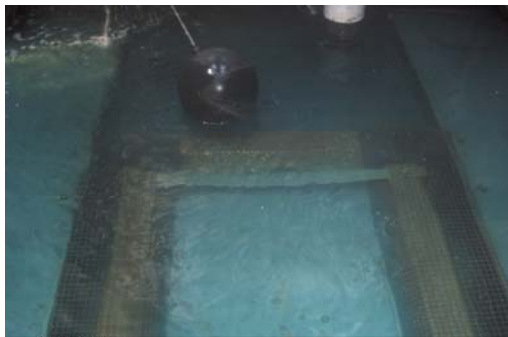
Scale Free Cooling Tower Basin
