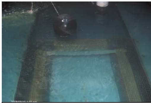
Scale Free Cooling Tower Basin
