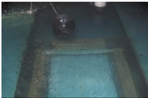
Scale Free Cooling Tower Basin
