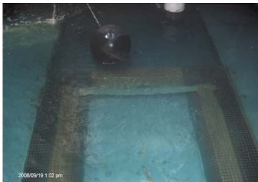
Scale Free Cooling Tower Basin
