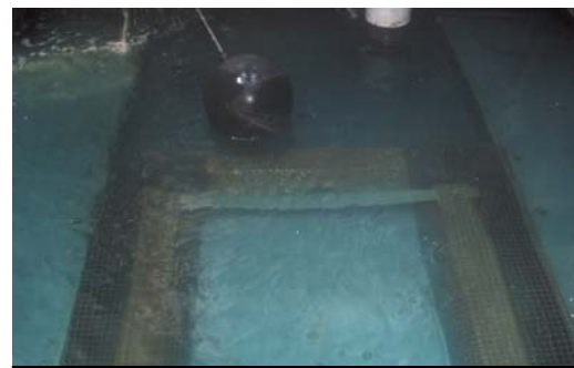
Scale Free Cooling Tower Basin
