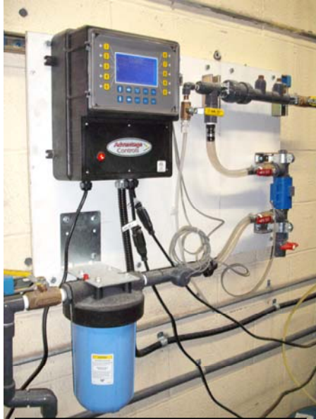
Installed BlueTrak Control
