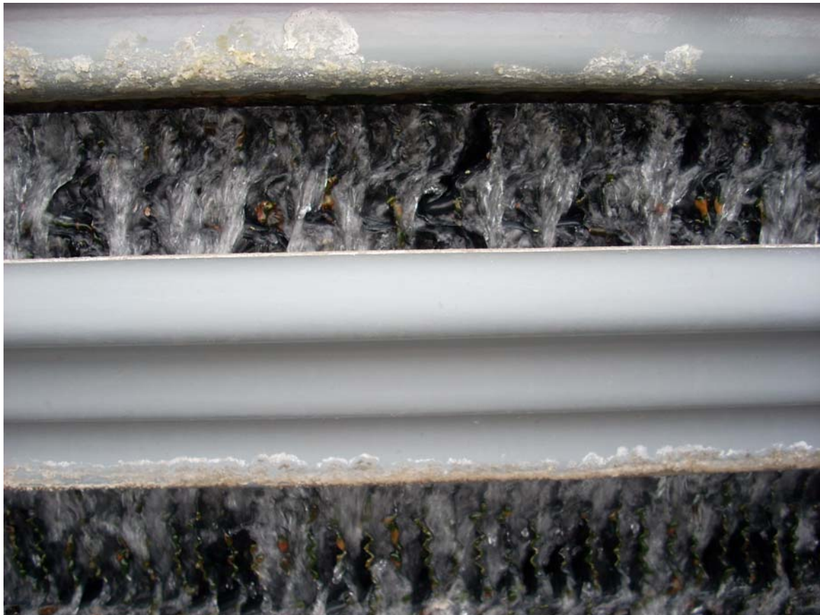
CT #2 fill showing algae growth on the fill.
